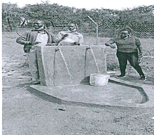
Figure 5: Newly Upgraded Lokitonyala Borehole
