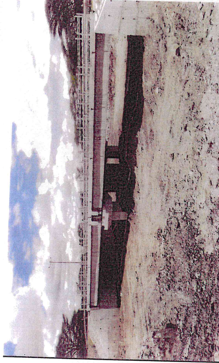
Widened 30m long two span concrete bridge at Km 36+093 along Kiserian – Isinya project corridor
