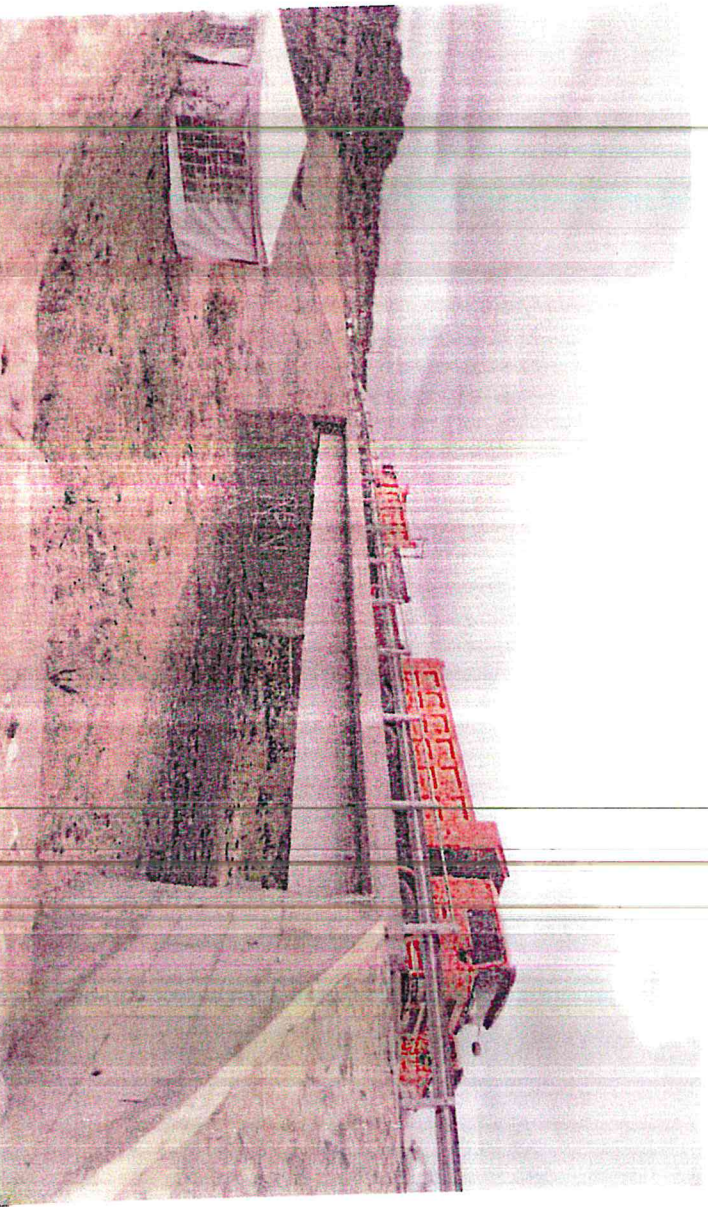
New 20m long single span concrete bridge at KM 17+757 along Kiserian – Isinya project Corridor
