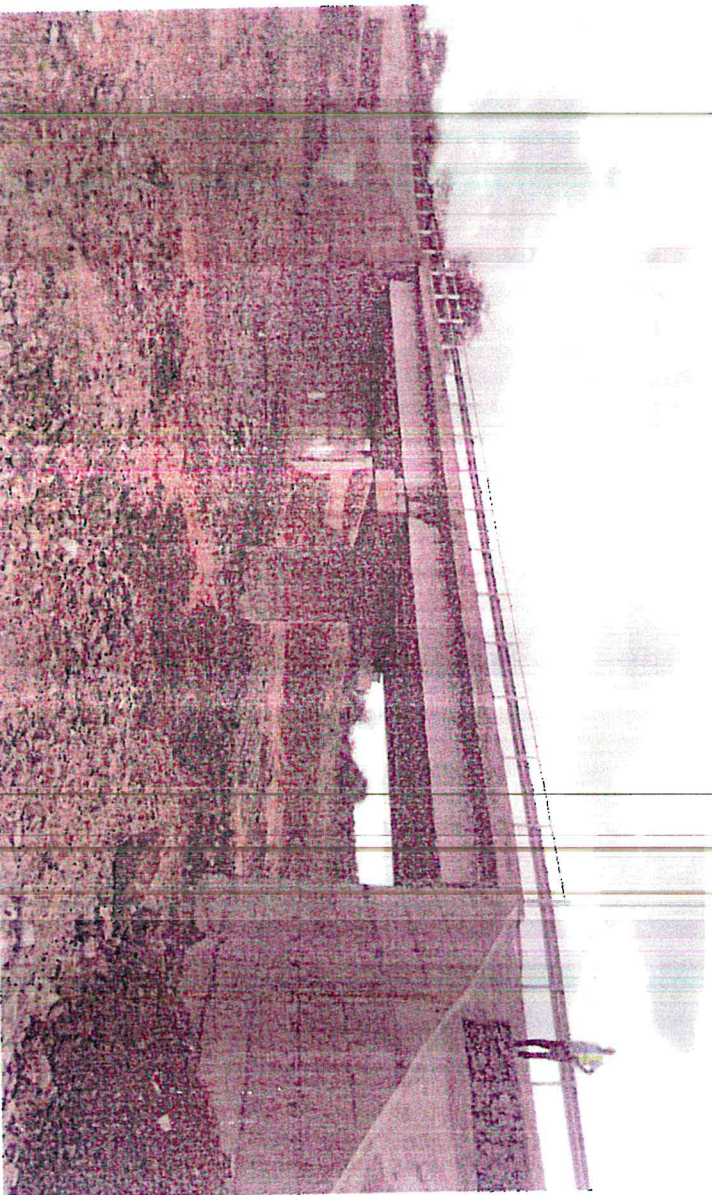
New 32m long two span concrete bridge at KM 32+777 along Kajijado – Imaroro project corridor
