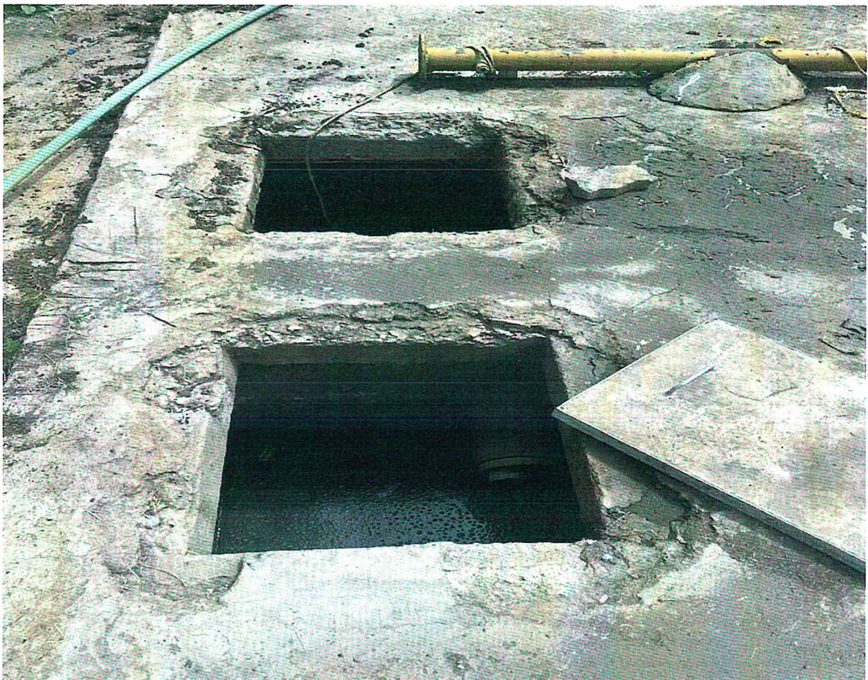
Figure 3. A dysfunctional ETP with open lids managed by MAVWASCO in Mavoko area
