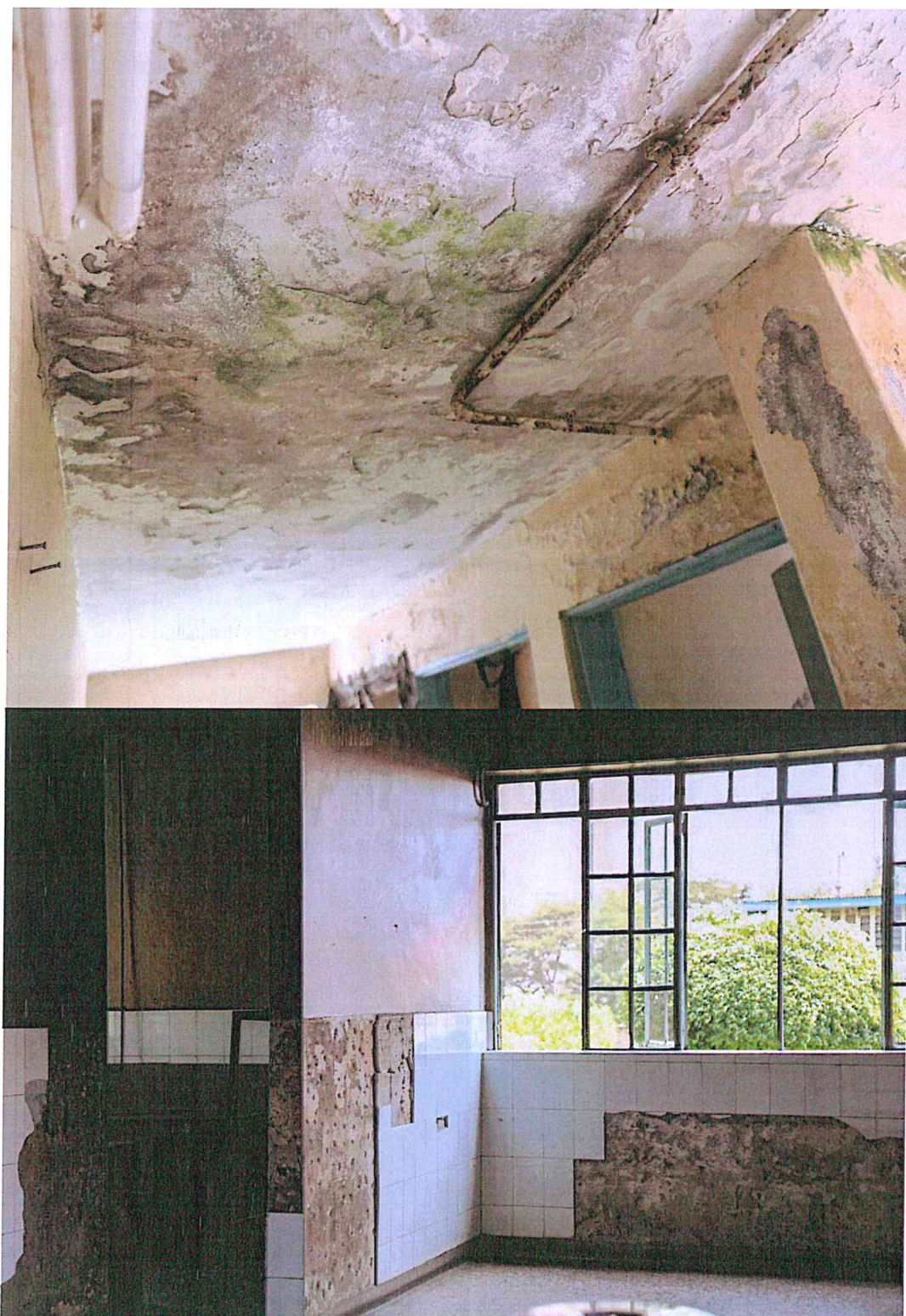
Picture 5 & 6: Severely damp and mould-infested corridor ceiling with corroded exposed pipework, highlighting chronic water leakage and poor maintenance and smoke-stained kitchen wall with extensive tile loss and exposed, deteriorated plaster demonstrating longstanding neglect of basic maintenance in the kitchen.
