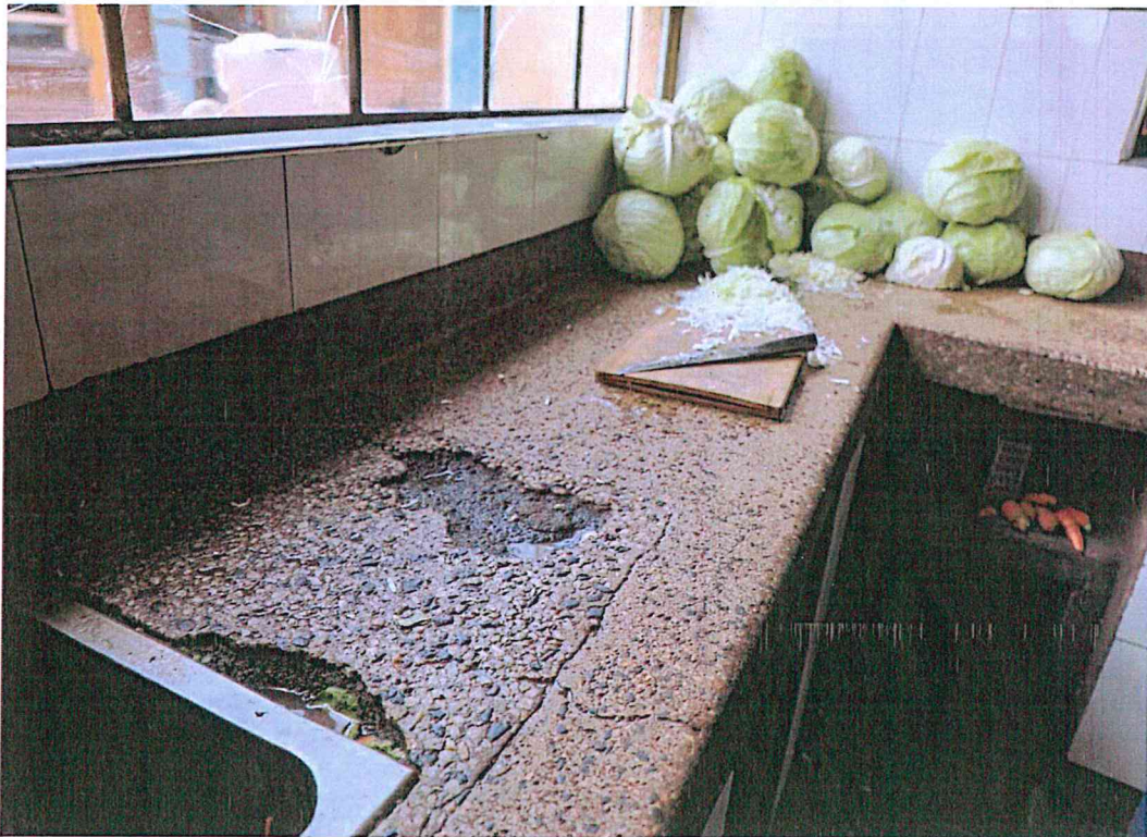
Picture 8: Severely worn kitchen worktop with potholes, stagnant wastewater and cracked surface where vegetables are being prepared, illustrating poor food-handling and infection-prevention standards.
