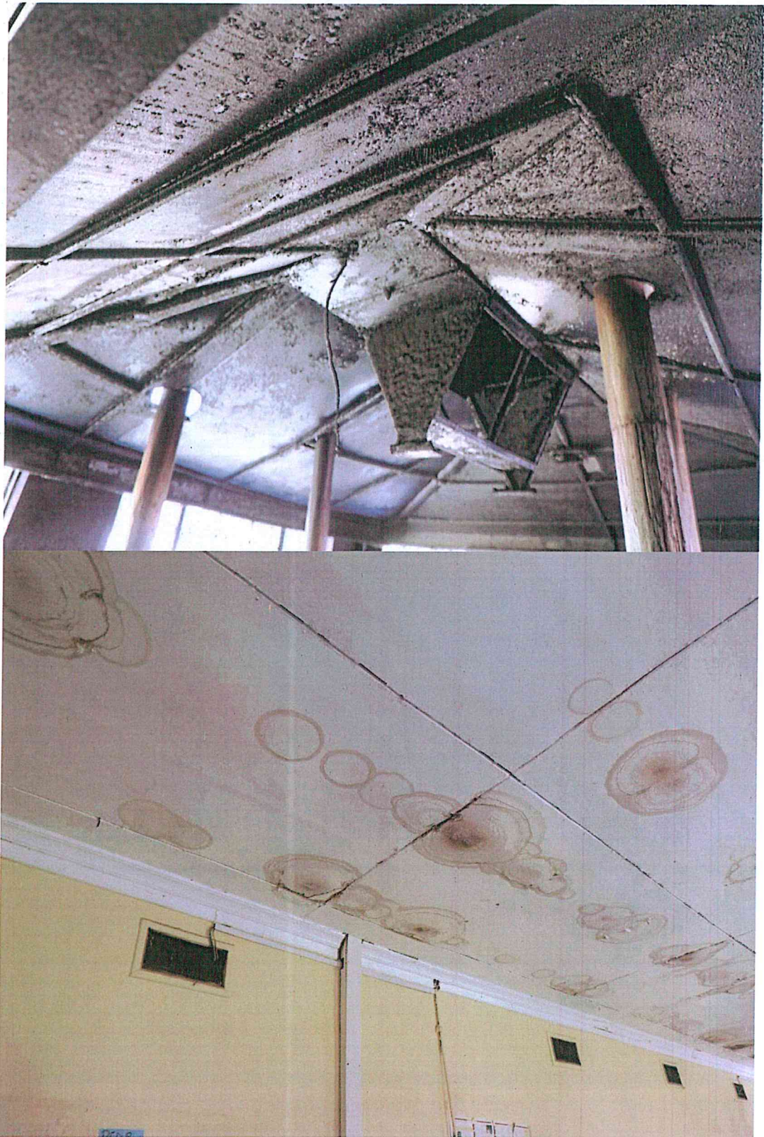
Picture 3 & 4 Damaged roof at Bungoma County Referral Hospital with damaged ceilings and loose electrical wires.
