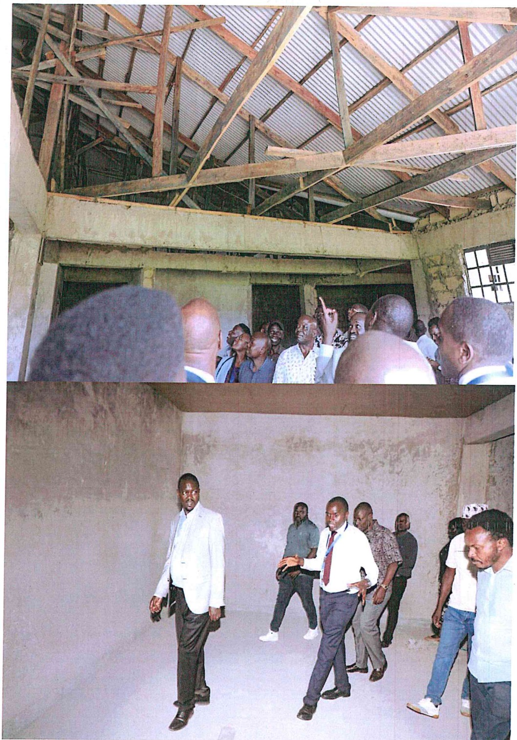
Picture 19: Internal view of the Radiography Complex under construction at Bungoma County Referral Hospital, where the Committee expressed concern over the poor workmanship.
