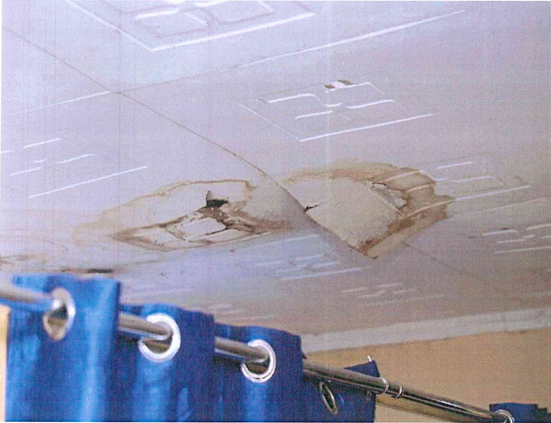
Picture 25: Ceiling damage at Kimaeti Health Centre with visible water stains, cracks and structural deterioration.
