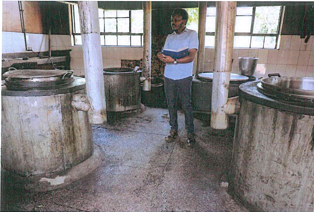
Picture 9: Old firewood-fueled hospital kitchen with large, soot-stained cooking pots and wet, slippery floor, highlighting outdated equipment and significant occupational and food-hygiene risks.
