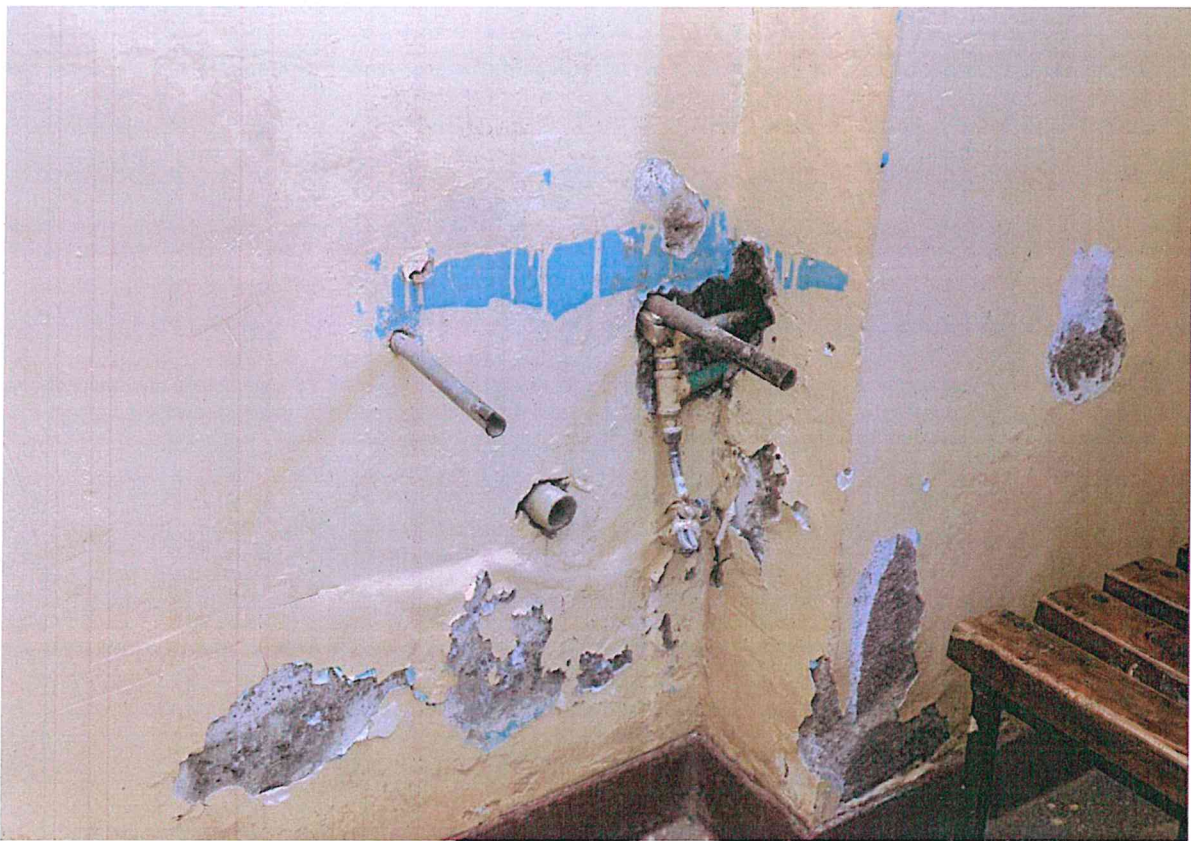
Picture 33: A section of dilapidated infrastructure at Kakamega County Referral Hospital.
