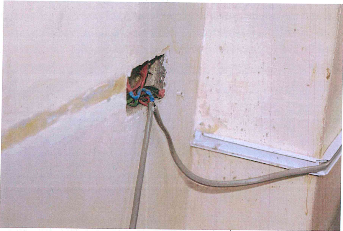
Picture 31: Exposed and poorly secured electrical wiring at Kakamega County Referral Hospital.
