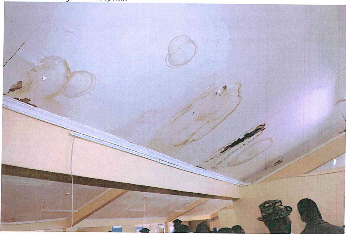
Picture 32: The water-damaged and deteriorating ceiling at Kakamega County Referral Hospital.
