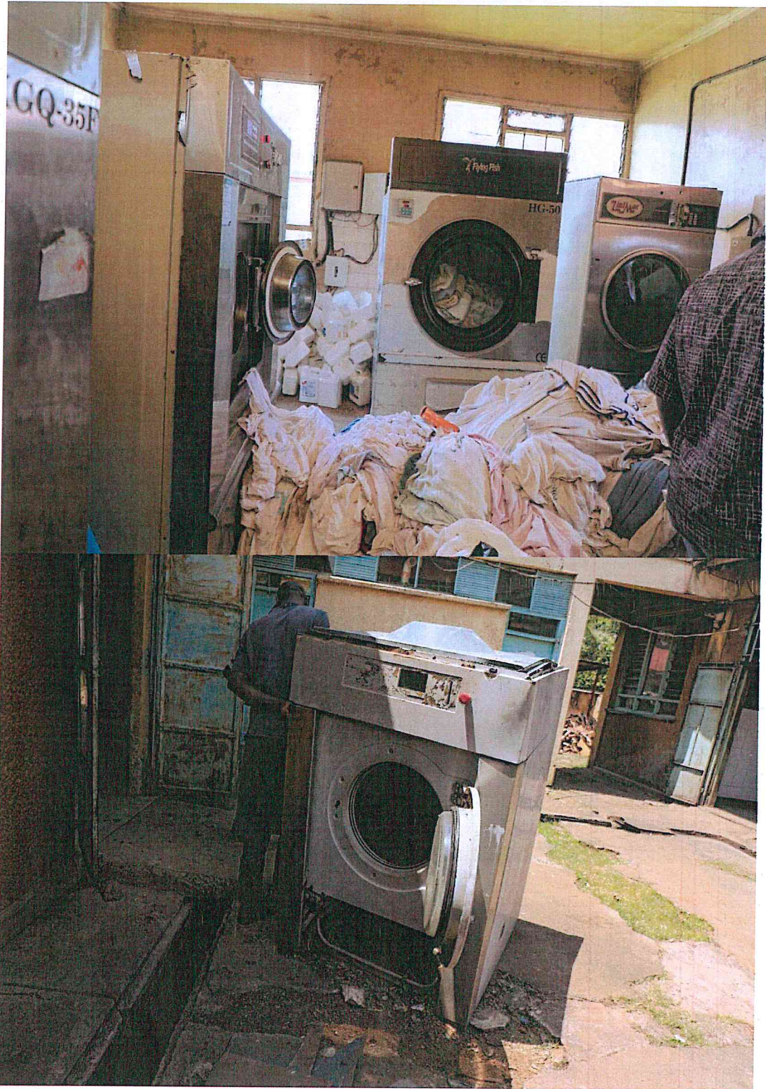
Picture 13 & 14: Congested hospital laundry room with ageing industrial machines and a heap of soiled linen on the floor and an abandoned washing machine lying outside the laundry section, symbolizing reflecting inadequate workflow, poor hygiene and limited capacity for safe linen management.
