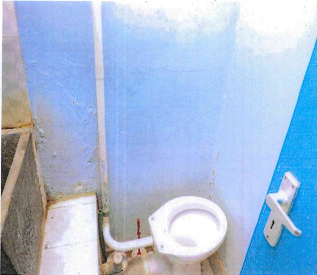
Picture 9: The bathrooms at the Hospital were dilapidated with visible cracks, peeling paints on the wall and signs of prolonged water damage on the walls and floor suggesting poor maintainance.
