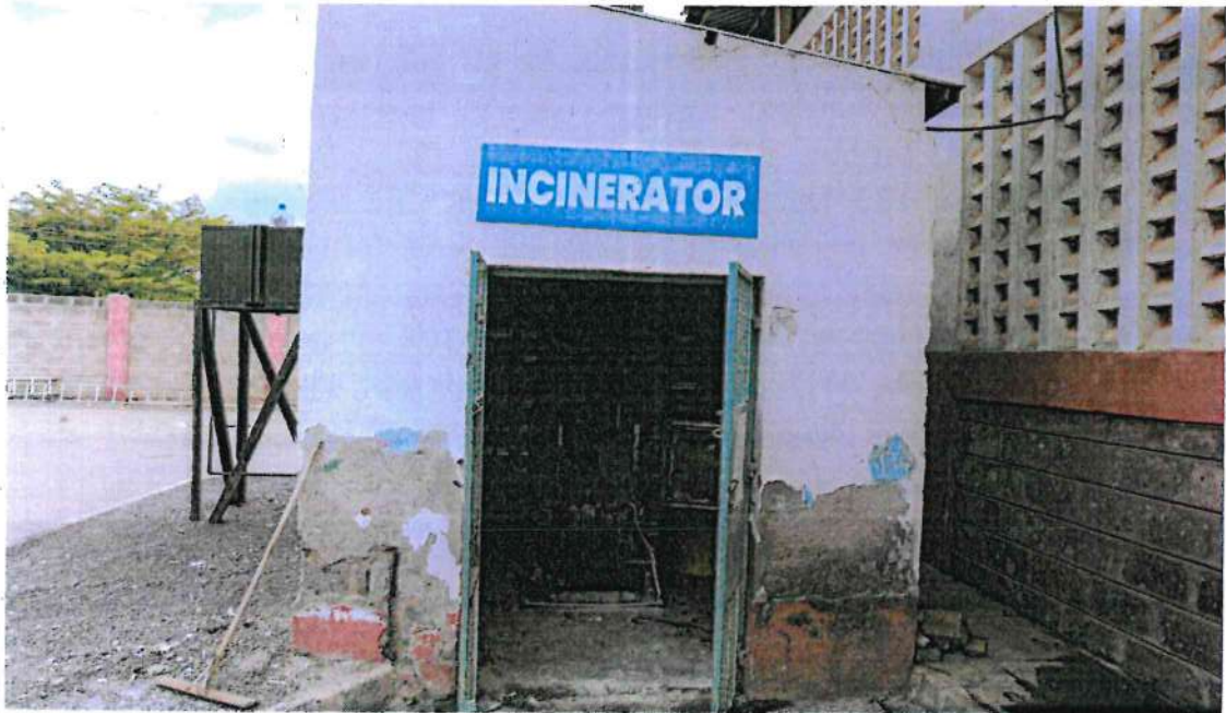
Picture 30: The incinerator at Machakos County Referral Hospital which does not have a functional entrance door.
