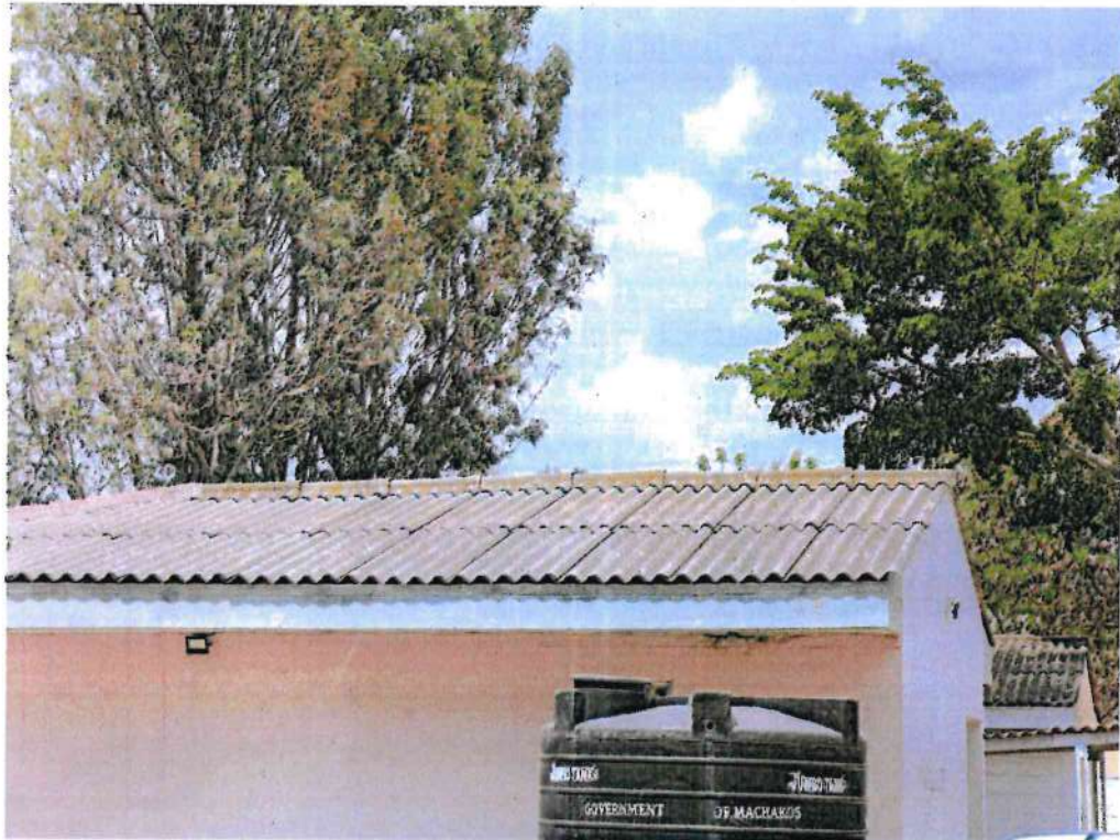
Picture 27: A roof with asbestos at the Mwala Level 4 Hospital which is scheduled to be removed and disposed before the end of the 2024/2025 Financial Year.
