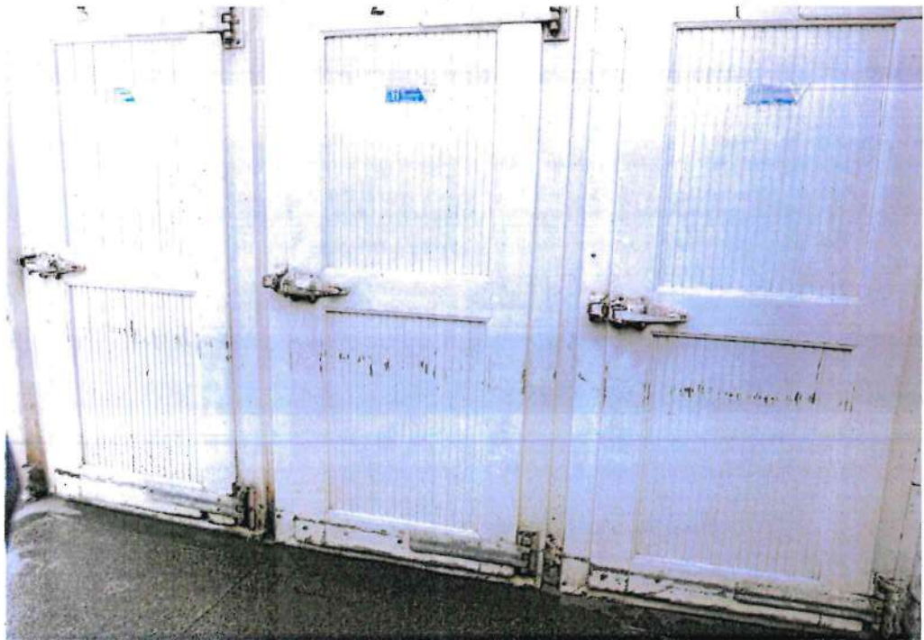
Picture 13 and 14: The dilapidated mortuary infrastructure at the Makueni County Referral Hospital.
