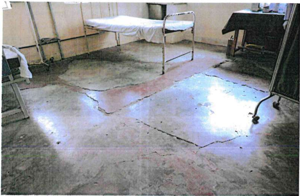
Picture 22: A Ward at the Athi River Level 4 Hospital face with poor physical infrastructure conditions including cracked floors.
