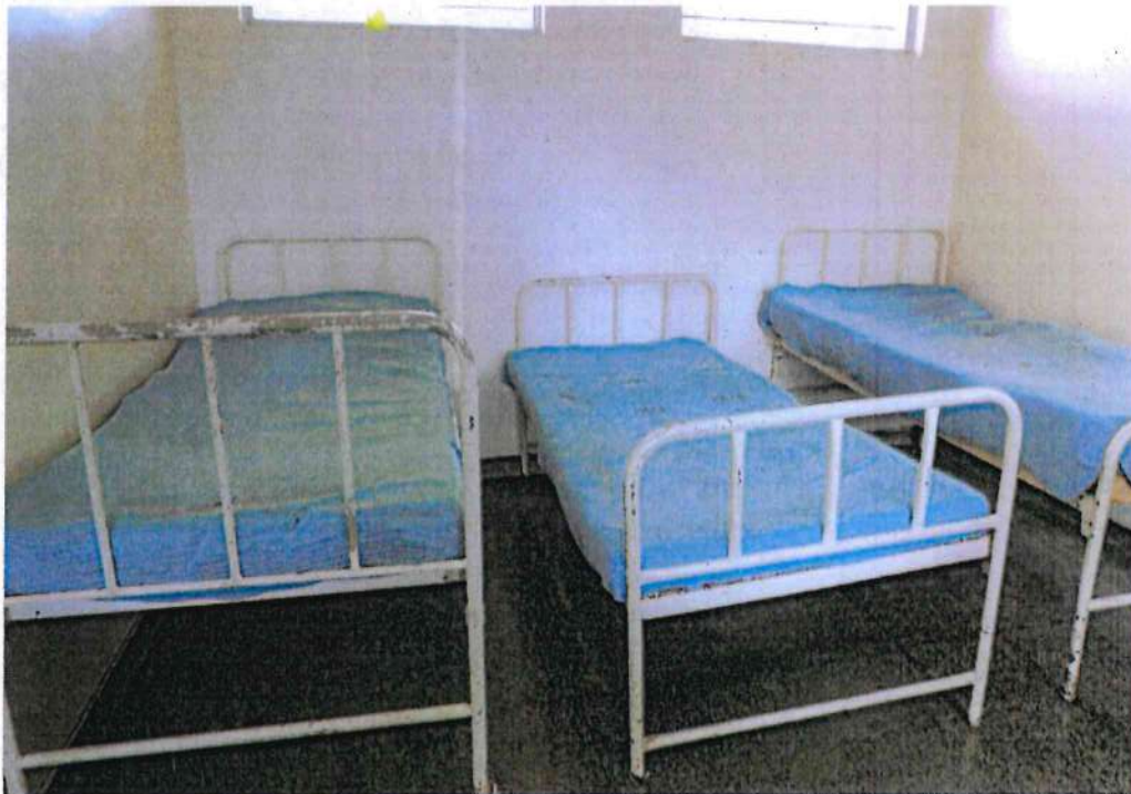
Picture 32: The rusty beds at the mental health unit.
