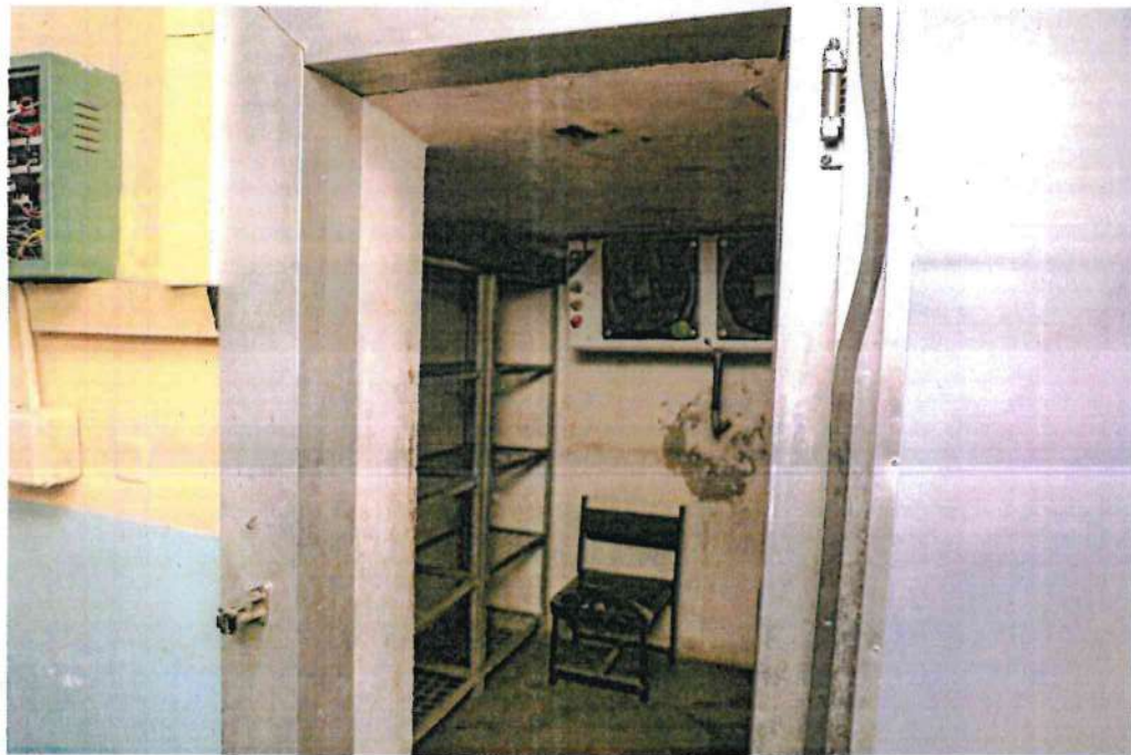
Picture 17: The Makueni County Referral Hospital kitchen was dilapidated as characterized by cracked flooring and unfunctional cold room.
