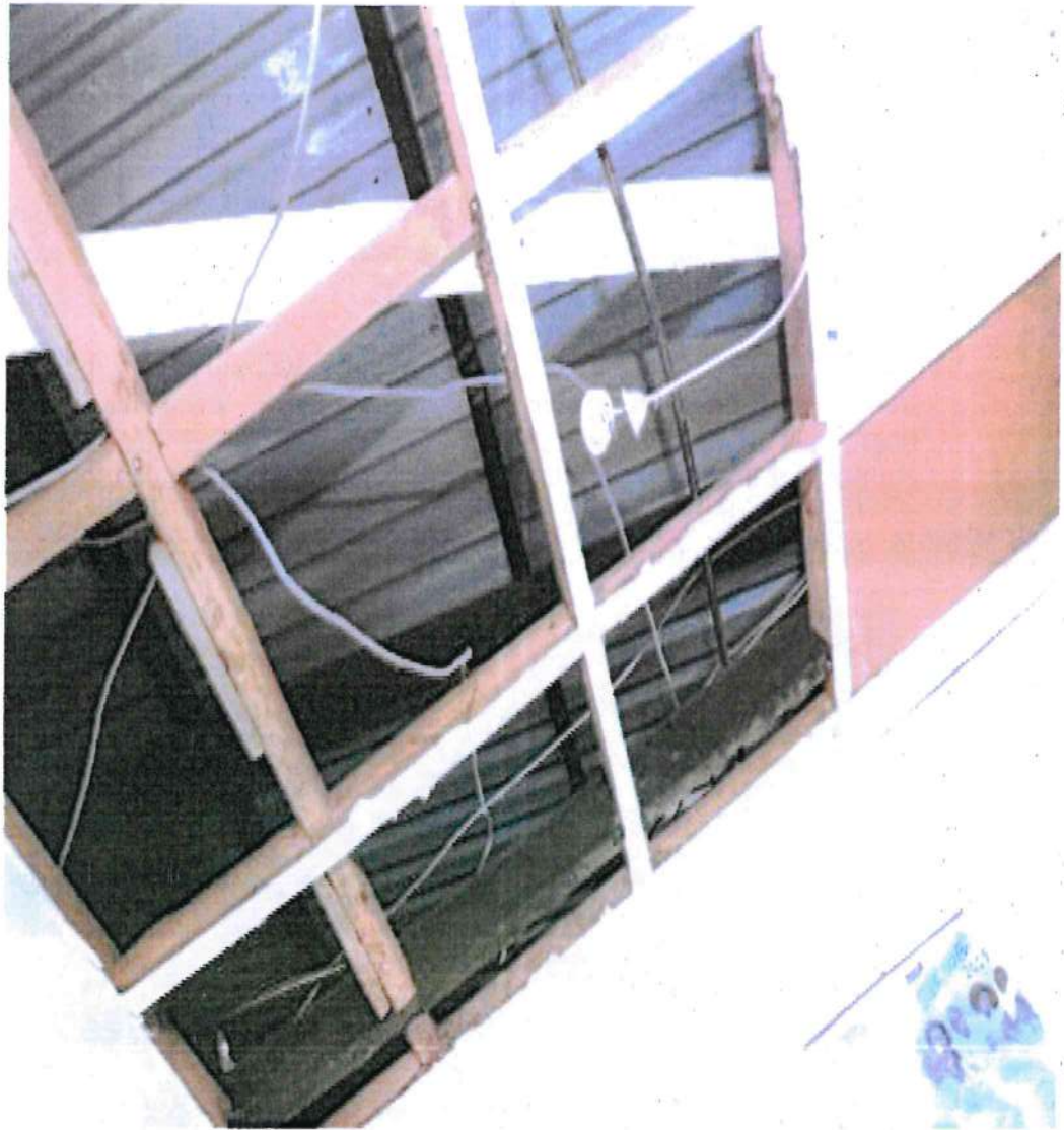
Picture 8: The section of the ceiling at Kitui Referral Hospital which had fallen off and ceiling panels are missing, exposing the internal framework, wooden beams, electrical wiring and the underlying metal roofing sheets.
